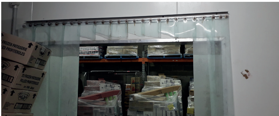
10. Strips cut off by staff to make access easier but resulting in no thermal barrier
