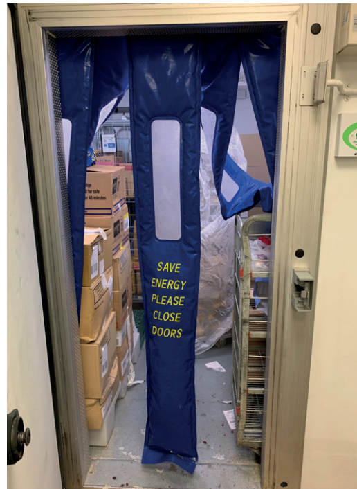
4. Strip curtains not forming a barrier
